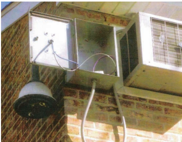
Lowden Homes Inoperable Security Camera
